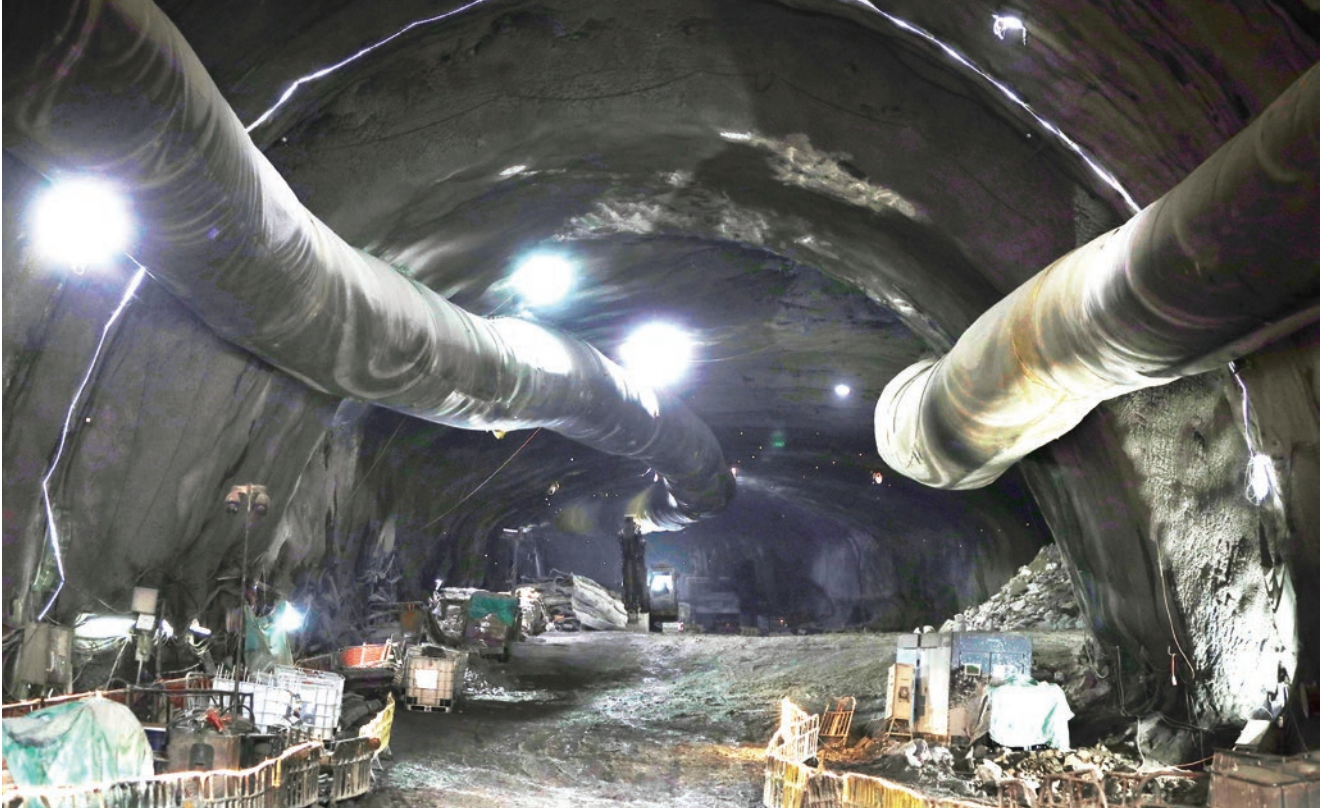
■ 2021年，政府便開始計劃把沙田污水處理廠搬遷到亞公角女婆山岩洞，是目前最大的岩洞發展計劃 In 2021, the Government began planning to relocate the Sha Tin Sewage Treatment Works to the cavern site at Nui Po Shan of A Kung Kok, which is currently the largest cavern development project in Hong Kong
